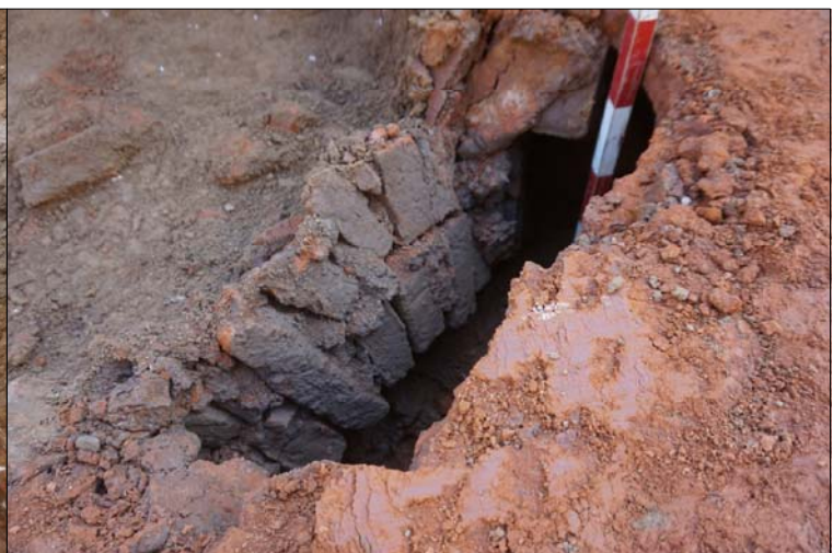
Looking north east at the collapsed arched ceiling of the kiln furnace tunnel
